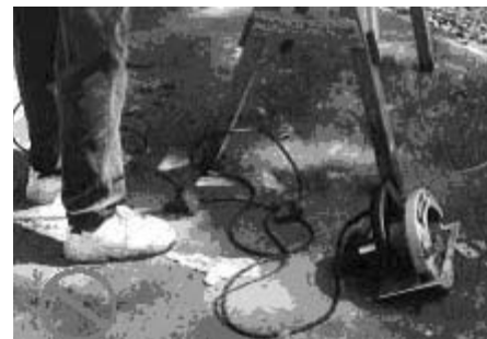
Combinations of hazards increase risk.
