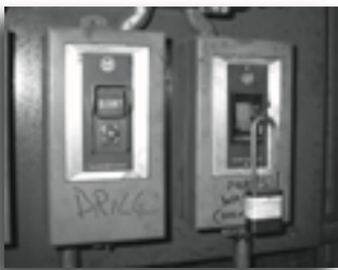
Main disconnect switch
